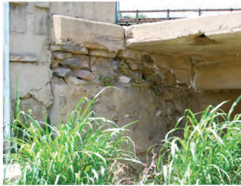
South abutment wall spall
