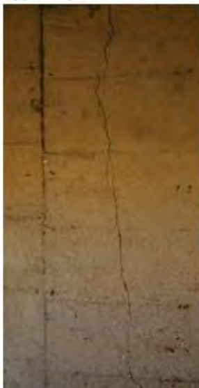
Typical pier vertical cracks
