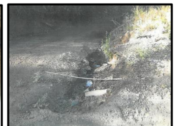
Erosion at the NW
