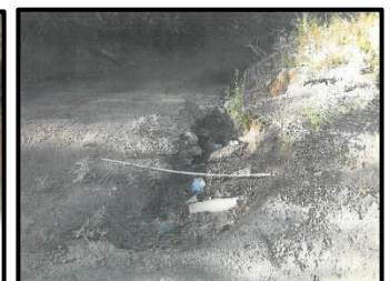
Erosion at the NW
