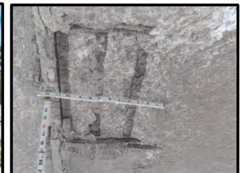
Large Spall in Soffit – Exposing Rebar
