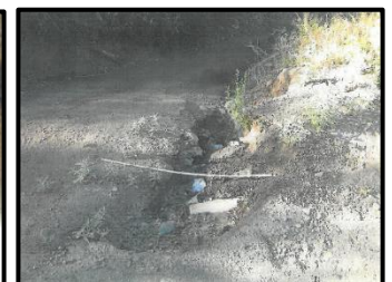
Erosion at the NW
