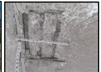
Large Spall in Soffit – Exposing Rebar
